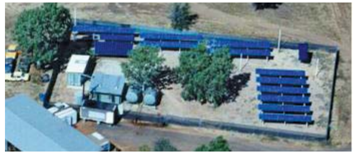
Figure 2. Photovoltaic array as part of a Hybrid Remote Area Power Supply at Jilkminggan in the Northern Territory of Australia. - Designed Constructed and Operated by the NT Power and Water
